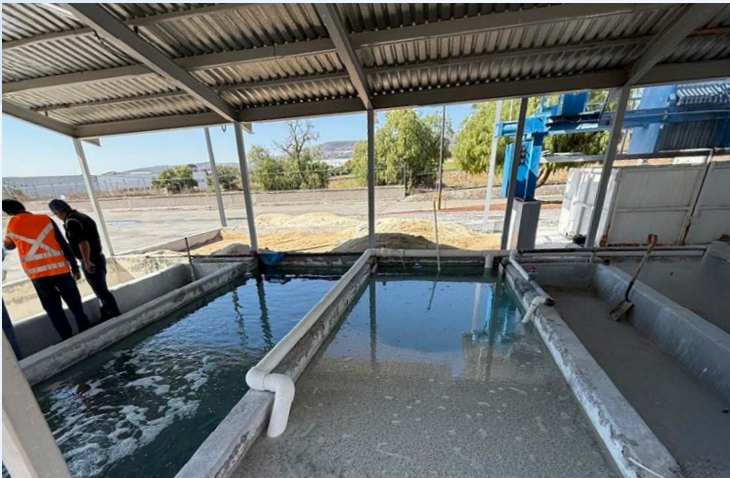
CCL Container Guanajuato, Mexico, On-Site Water Treatment System
