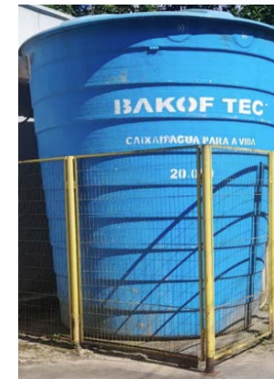
Checkpoint Brazil, Rainwater Capture Tank
